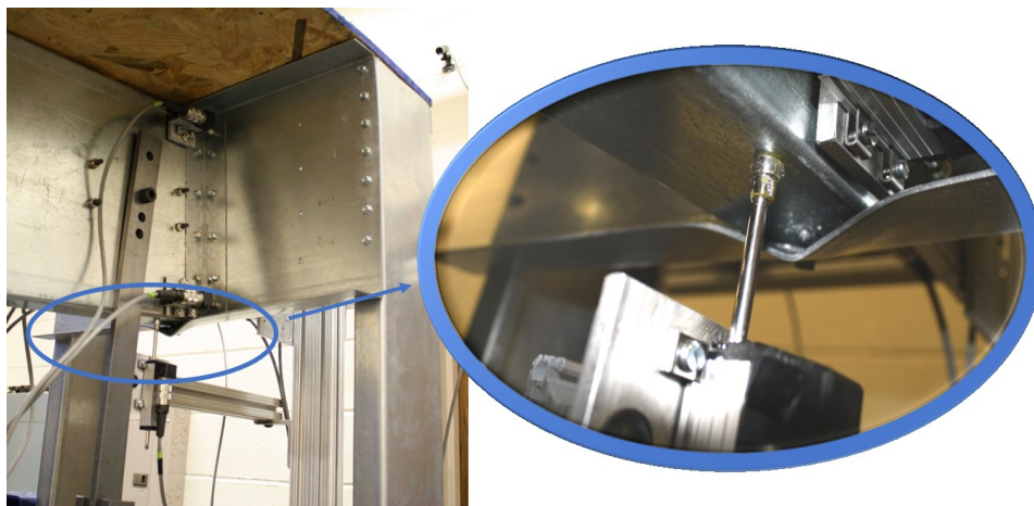
Figure 8: Screw failure at bottom ledger of the T25
